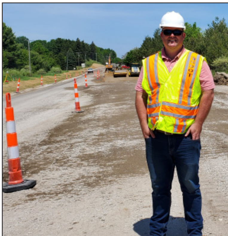
Garrett Dawe, MDOT service center manager in Alpena, talks about the $5 million road construction project that began April 15. Photo by Cheryl Peterson.
