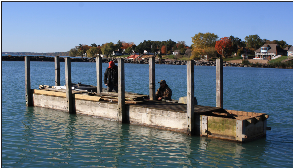
Workers float a finger dock from the harbor to the DNR boat launch.
