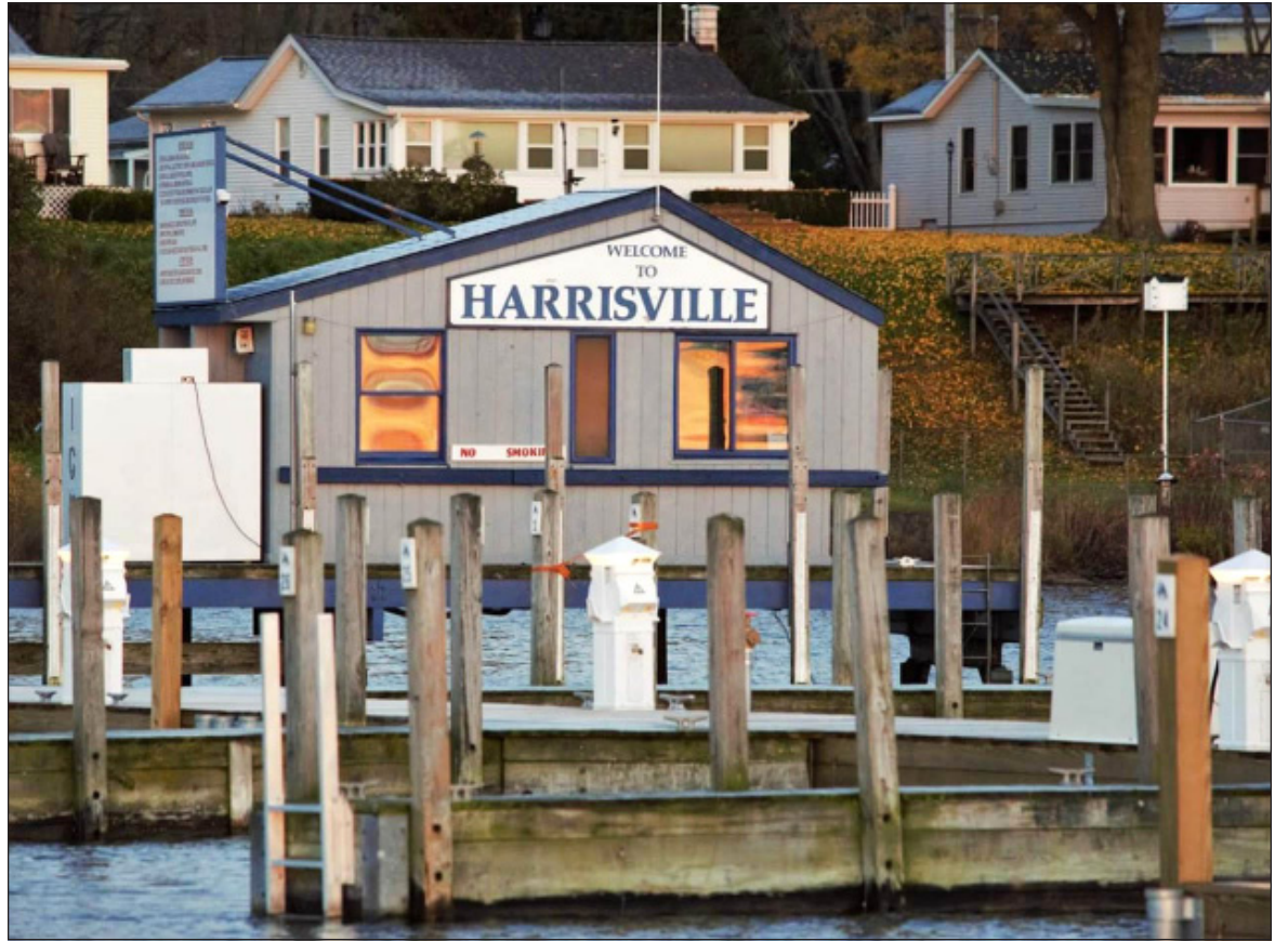
The iconic gas shack at Harrisville Harbor is no more. It was torn down last week as part of an on-going improvement project. A new gas shack will be constructed in the same footprint with a similar design. Photo courtesy of Jim Ferguson.
