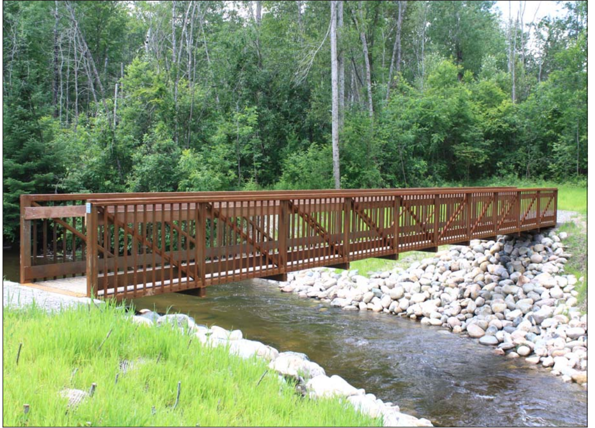
The new pedestrian footbridge which connects pathways to large tracts of land within the Huron Manistee National Forest over the South Branch of Pine River is in place and the old Buhl Dam, which had been obsolete for several decades and impeded the water flow has been removed. Photo by Mary Weber.
