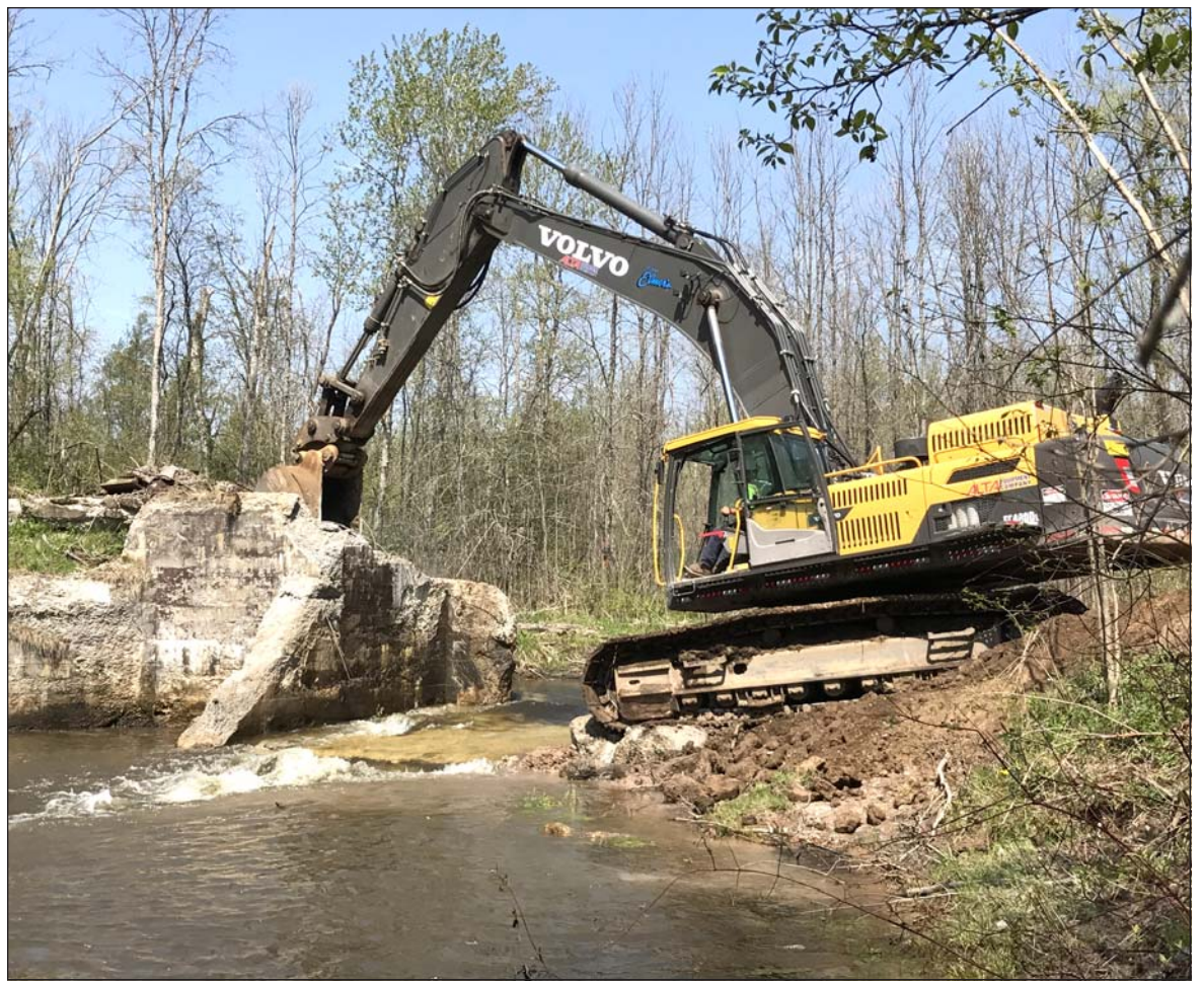
Team Elmers, contractor for the demolition of Buhl Dam, work carefully, but efficiently, during the removal process. Courtesy photo.
