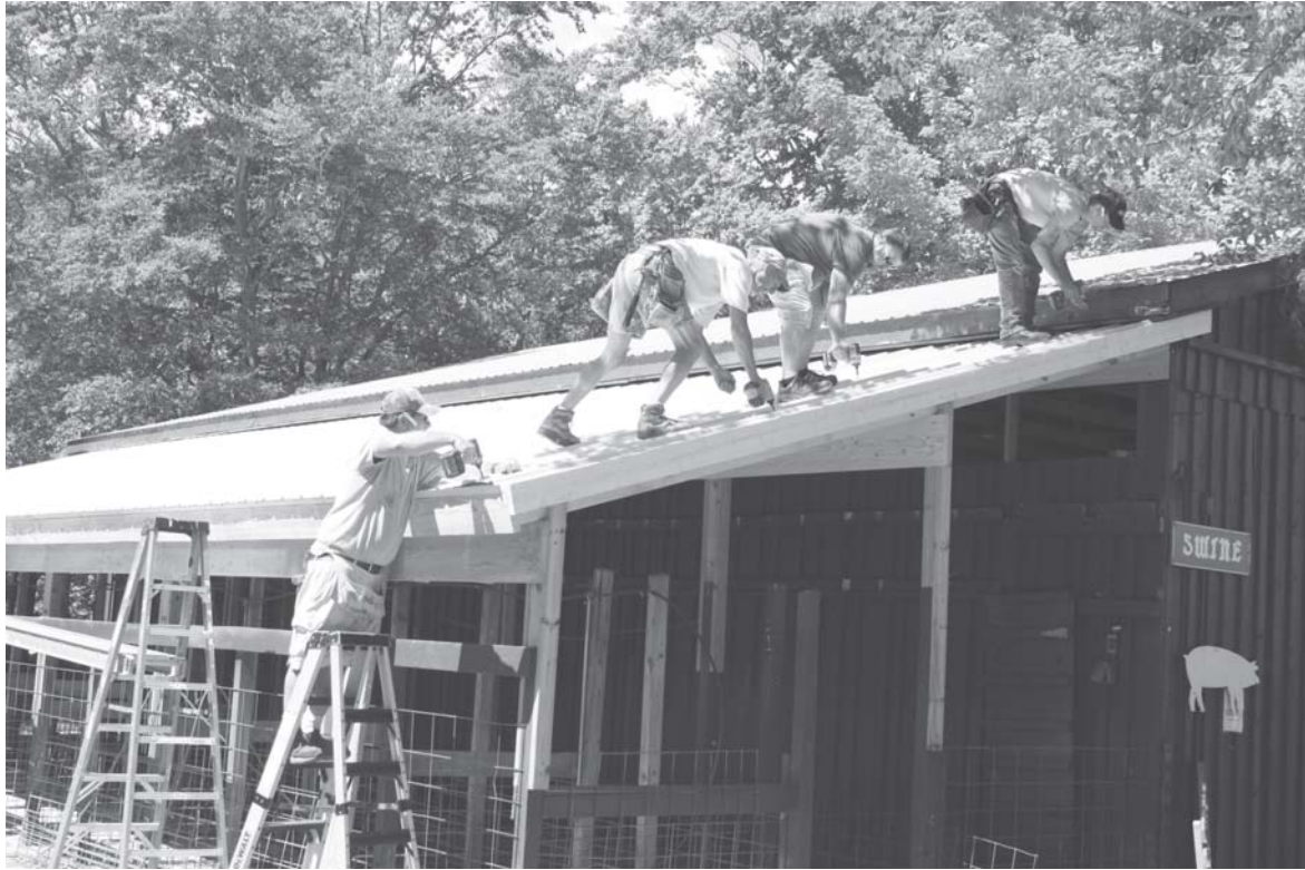
Volunteers (from left) Tommy Jacobs of Jacobs Construction and his crew, Jason Livingston, John Pfantz, and Doug Mullin, finish the new roof on the pig barn at the Alcona County Fairgrounds. The raised roof will allow better ventilation to keep swine diseases down. Doorways were also raised on the barn. Photo by Willy Weber.
