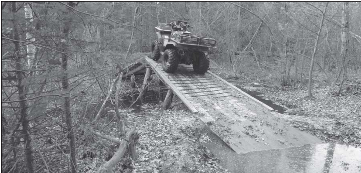
Work is taking place in this photo to construct a deck over a watery area in the Lower Peninsula.
