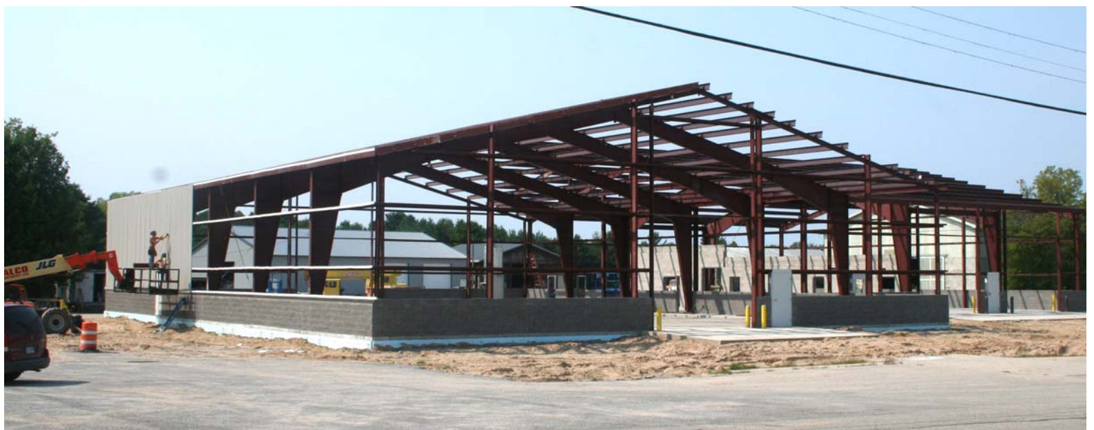
The exterior shell of the new Alcona County Road Commission building in Lincoln is being put up this week. According to Jesse Campbell, the past two weeks have shown quite a bit of progress. "All is going well; we are still looking to be completed by November 1," Campbell said. "We still have a ways to go... the building is going up fast, but time seems to be going faster." Photo by Cheryl Peterson.
