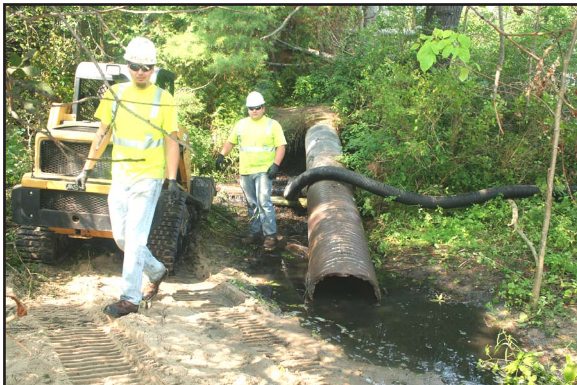
Employees of City Sewer Cleanup on site Tuesday work to clean up the residue from the raw sewage leak into the City of Harrisville's storm sewer system. Photo by Cheryl Peterson.
