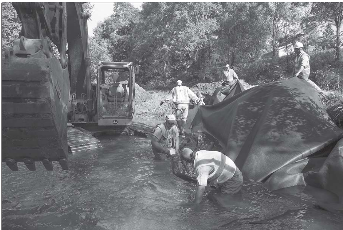
Michigan DNR workers join contractors in Highbank Creek during a stream-restoration project. Photos courtesy of Michigan DNR.
