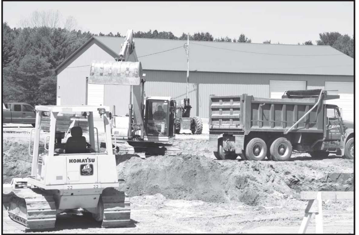
Work on the site of the new road commission garage began last week. Once the density tests are completed and no problems arise, footings will go in for the 17,000 square foot building. Photo by Kirk Walton.
