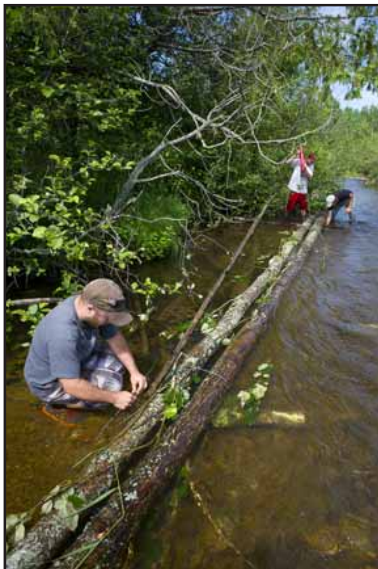
Members of the Upper Black River Council help place structure to improve trout habitat on the upper Black River in the northeastern Lower Peninsula.
