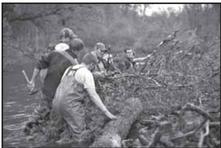
Workers arrange woody debris in the North Branch of the Au Sable River. Photos courtesy of Michigan DNR.
