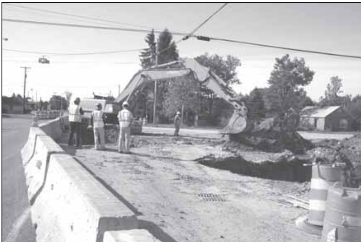
The road barriers and detour are in place and soil removal is underway in Mikado at the corner of F-30 and F-41. The project, which began roughly two weeks ago, will be ongoing until early October. The Michigan Department of Environmental Quality (DEQ) identified the contaminated site in 2008. The project is being funded by federal dollars. Photo by Cheryl Peterson.
