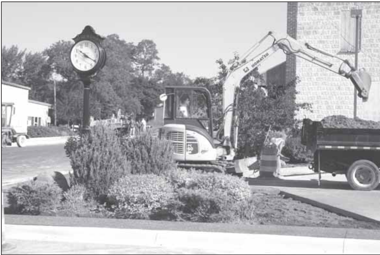
Phase One of the streetscape project in the Village of Lincoln is nearing completion. According to village president Phillip Jordan, the last layer of pavement will be put down this week and finishing touches are being put on the sidewalks and some of the landscaping (above). Lights will be placed in September and trees will be planted after the lights are put in. Finishing touches are just in time for the 13th Annual Lincoln Lions Antique and Classic Car and Tractor Show which will be held on Second Street Saturday. For more details see pages 10 and 11. Photo by Cheryl Peterson.
