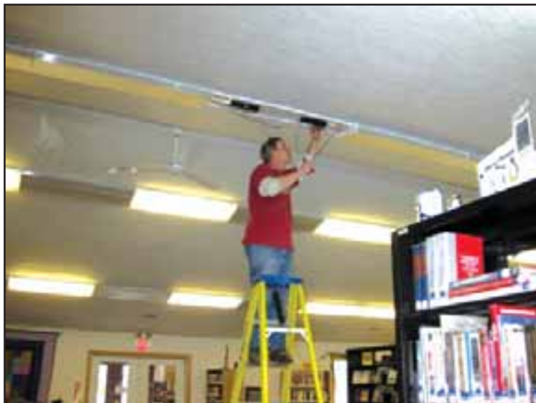
George Schultz, Curtis Township Library maintenance engineer, is replacing 56 ballasts at the library in conjunction with the new energy saving lights through a Consumer's Energy Incentive. This incentive program is available to businesses that want to replace their T12 lights and ballasts with the more energy efficient T5/T8 lights and ballasts. The library decided to keep existing fixtures and replace the ballasts and lights. Incentives from Consumers will cover the entire cost of the new T8 ballasts. The library's only expense are the new T8 bulbs, which are approximately $350. The project began April 1 and is expected to be completed by April 23. The incentive can be found at www.consumersenergy.com , search under business energy efficient programs for the "lighting retrofit incentives worksheet." Courtesy photo.
