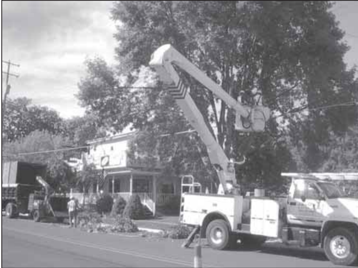
Work crews from J. Ranck Electrical, Inc. remove trees in front of The Old Place Inn in downtown Harrisville Monday. Tree removal and tearing up the old sidewalk began last week. Photo by Art Kniep.
