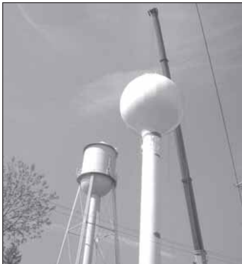
A crane places the water storage tank atop the new water tower. The new tower went up last Thursday and will be painted blue. Photo by Art Kniep.
